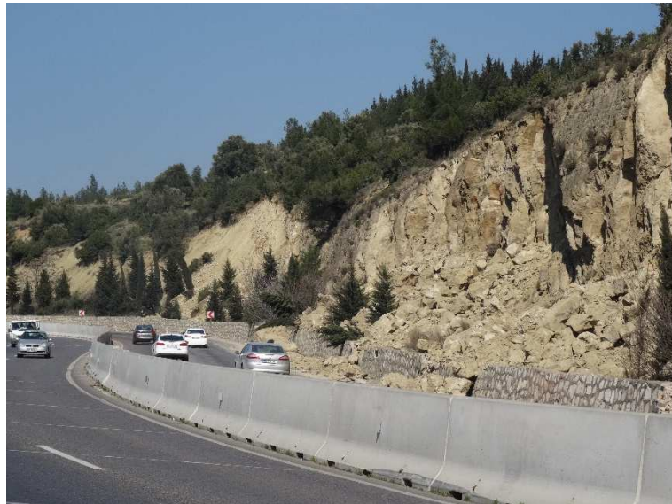
Figure 3. Rockfalls triggered in sandstones by 6 th February Kahramanmaraş earthquakes along Hatay – Belen highway.
